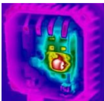
Figure 36 - Surchauffe d'une diode bypass
